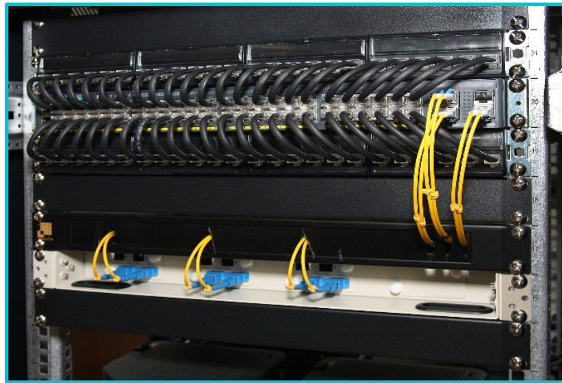
Patch panel with ethernet cables
